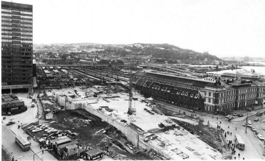
Oslo-tunnelen under bygging, sett fra sentrumssiden (september 1977). The Oslo Tunnel under construction, view from the city centre (September 1977).
