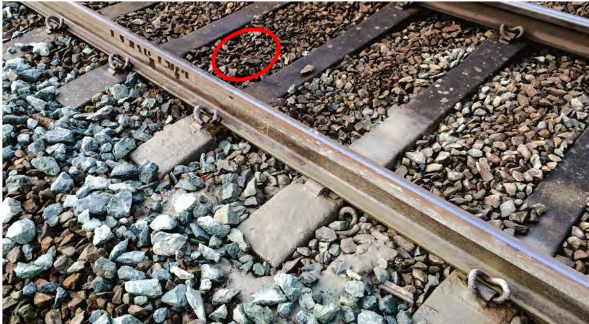
Figure 29: Water test site 2. Fines from mud pumping clearly visible on sleeper ends and adjacent ballast. Water was poured into the area marked in red.
