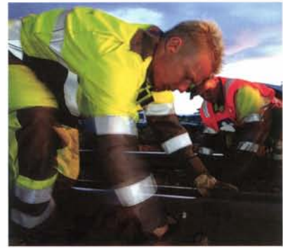
Track maintenance technician Arild Kvaal works on a track switch, while Vegard Lade acts as lookout. Photo: Øystein Grue
