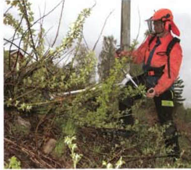
Clearing vegetation at Bleiken station on the Gjøvik line. Photo: Njål Svingheim
