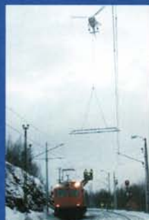
April Jernbaneverket saves time and money by using a helicopter to install overhead line equipment on the Ofoten line. Photo: Carl Næsje, Fremover
