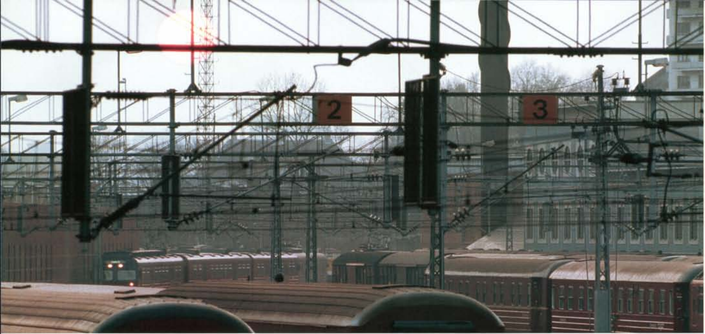
The catenary has to be renewed when lines are upgraded for speeds of 160 km/h upwards. (Photo: Rune Fossum)
