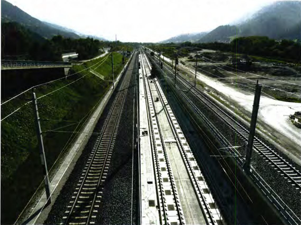
Figure 169. Construction of the new feeder line to the Brenner base tunnel – “Unterinntalbahnhof”. Big construction sites were needed which had an influence on large areas, shown to the right in the picture.
