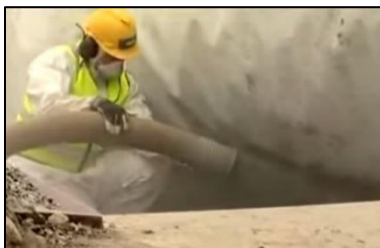
Figure 4.22 – Illustration: Soil blowing on the sides of Haugenstua pipe culvert in 2008 (Source: Gjermnudshaug Gruppen)
