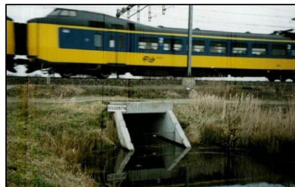
Figure 1.2 – Southern side of the box culvert during a train passage. The water table can be seen at surface level (From Hölscher. P and Meijers. P 2009)
