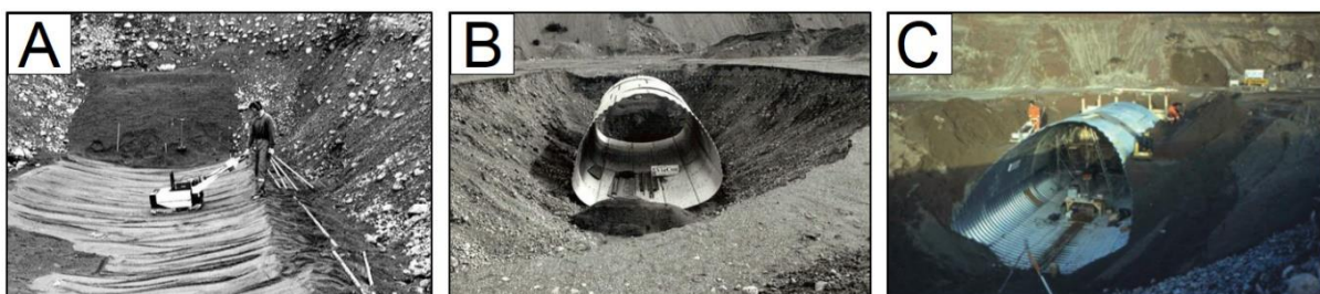
Figure 6.9 – Installation of the Enköping test culvert from Sweden in 1987, showing A) preparation of the foundation, B) installation of the culvert in the excavation pit and C) backfilling (Modified after Petterson, L, 2007)
