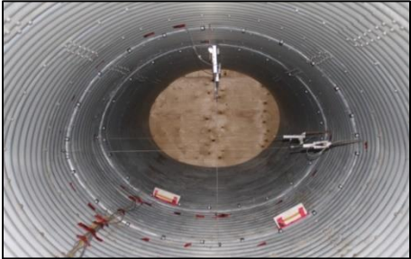
Figure 6.19 – Placing of fiber optic sensors cables and DIC targets (From Moore. I. D, 2017)
