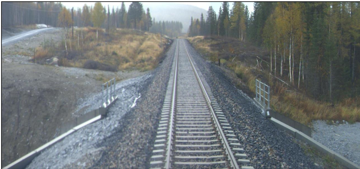
Figure 3.4 – ROGER 1000 photo before the measuring vehicle is passing Svenningdal culvert (Source: Bane NOR)
