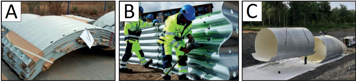
Figure 4.18 – The merging process of an SSCB, showing A) the steel plates delivered in bundles, B) bolting of the steel plates together in sections and C) sections being mounted together (Modified after Viacon, 2015)
