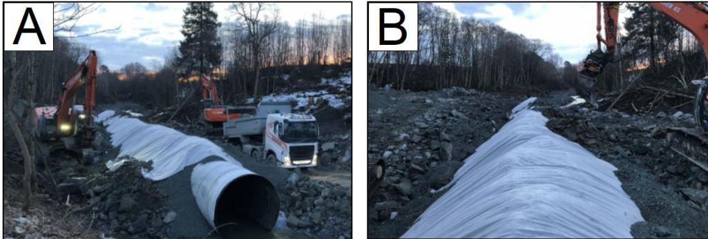
Figure 4.24 – Illustration: Using a non-woven geotextile as a separation medium for the upper top arch of a pipe, reducing the risk of materials from the inner and outer zone to mix (Source: Farbu & Gausen AS)
