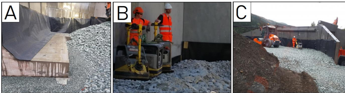
Figure 4.7 – Illustration: Backfilling and compaction during different steps of building of the Kilnes element culvert, showing A) the finer corrective layer underneath the culvert, B) a closeup of the 20/120 mm crushed rock material and C) how the compaction work is performed in the different zones (FOTO: Farbu & Gausen AS)
