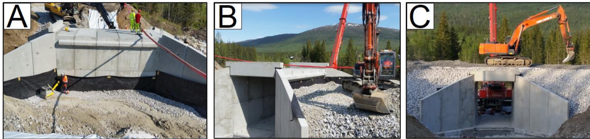
Figure 3.3 – Installation and backfilling of Svenningdal culvert in 2016, showing A) compaction work, B) when the backfill has reached the slab level and C) Overfilling (Source: Farbu & Gausen AS)
