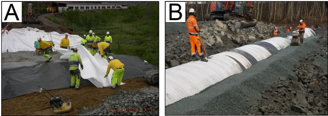
Figure 4.23 – Backfilling at A) Solheim culvert in 2009 and B) Ydsedal culvert in 2018. For case A) sand were used as the inner layer while for case B) a finer crushed rock were used. In both cases crushed rock ranging in between 20/120 mm were used for the outer zones (Source: Viacon Norway and Farbu & Gausen AS)
