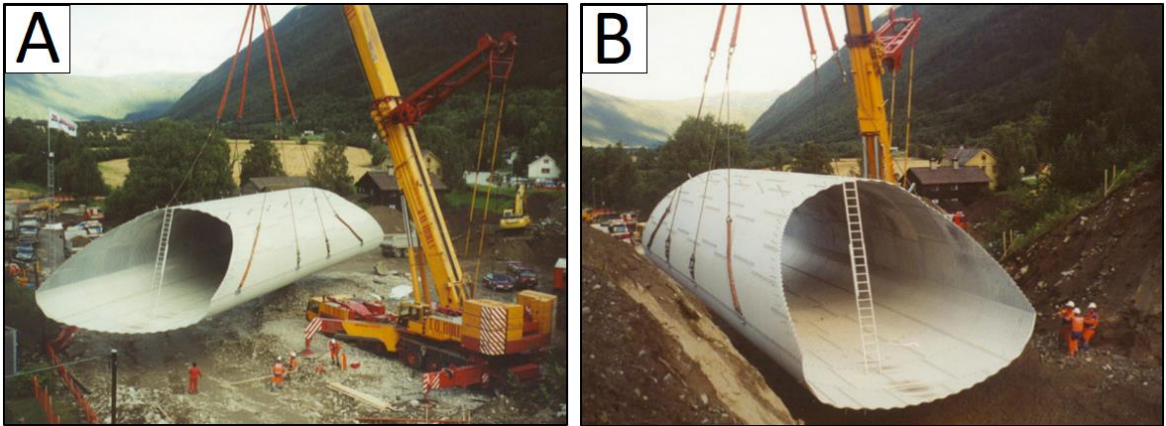
Figure 4.20 - Installation of Sel Fv. 438 pipe arch culvert in 2002 with a mobile crane under the Dovrebanen railway line. The culvert had a span length of 9.6 meter (Source: Jan Vaslestad)
