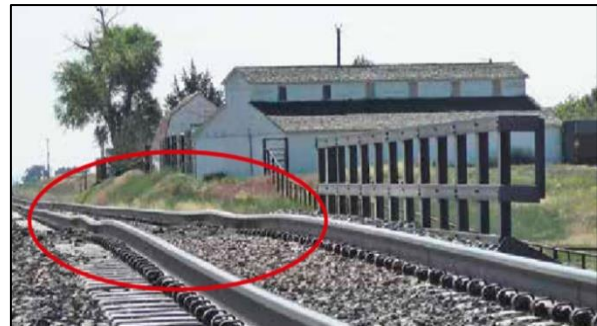
Figure 1.2 – Illustration: An extreme case of vertical track irregularities in the transition zone, clearly showing the characteristic «dip» before the bridge (Source: www.railwaygazette.com )
