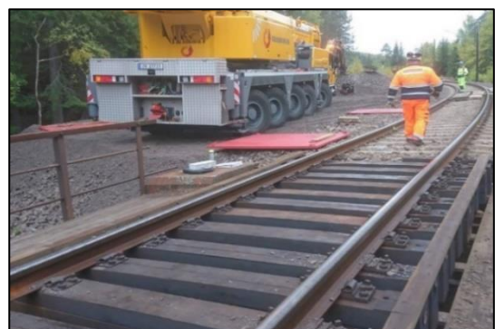
Figure 1.1 – Illustration of a fixed track: Trangrud railway bridge in Norway during reconstruction from fixed to ballasted track on the bridge with trough, autumn 2018 (Source: Rallar Service AS)
