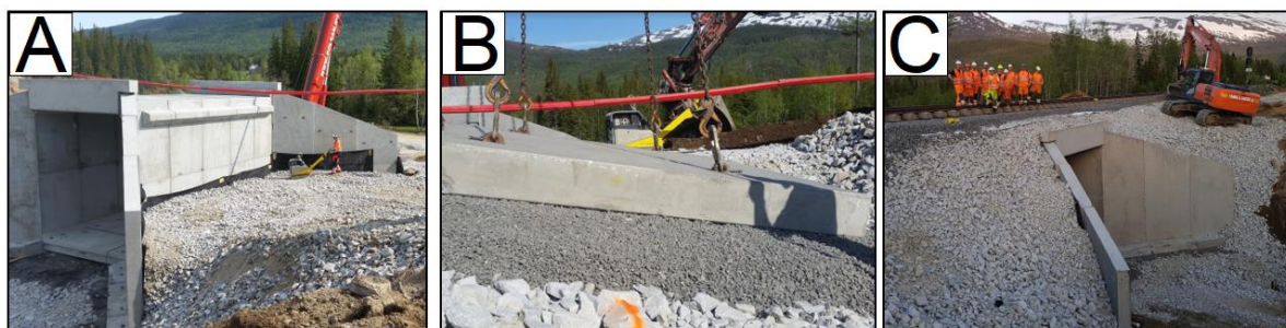
Figure 1.6 – Backfilling stages for Svenningdal culvert built in 2016, showing A) compacting a 20/120 mm crushed rock material with a light vibroplate, B) installation of the transition slab and C) construction finish (FOTO: Farbu & Gausen AS)
