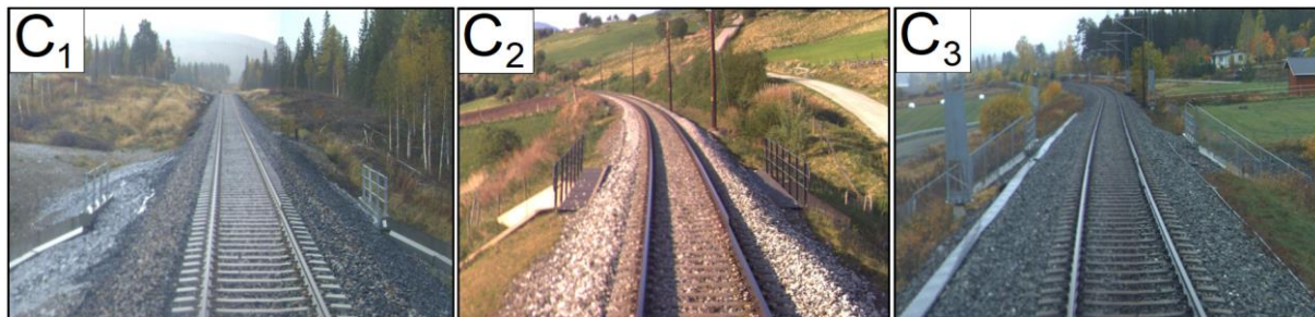
Figure 5.4 - ROGER 1000 photos showing site conditions at C 1 ) Svenningdal, C 2 ) Vinstradalsveien and C 3 ) Jarenhaugen culvert
