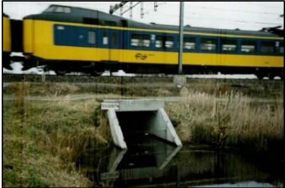
Figure 4.10 - The «Gouda Goverwelle» culvert during the passage of a passenger train (Modified after Hölischer, P, Meijers, P, 2009)
