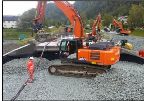
Figure 2.36 – Demonstration: Backfilling at Kilnes culvert from 2016, indicating that the material may be expected to be very rigid in relation to the culvert (FOTO: Farbu & Gausen AS)
