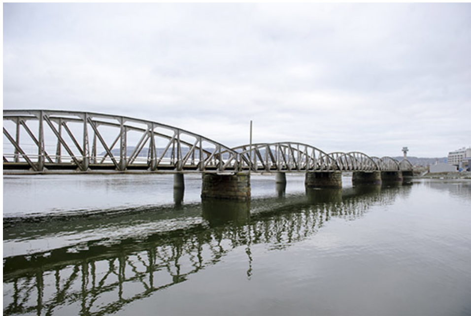
Figure 3.1: Hell Bridge when still in normal service.
