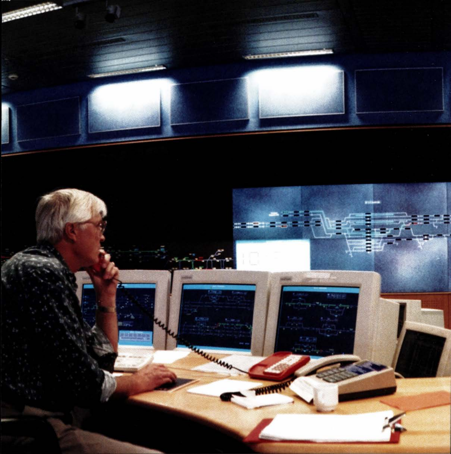
The entire Gardermobanen is controlled from the remote control centre at Oslo Central Station.
