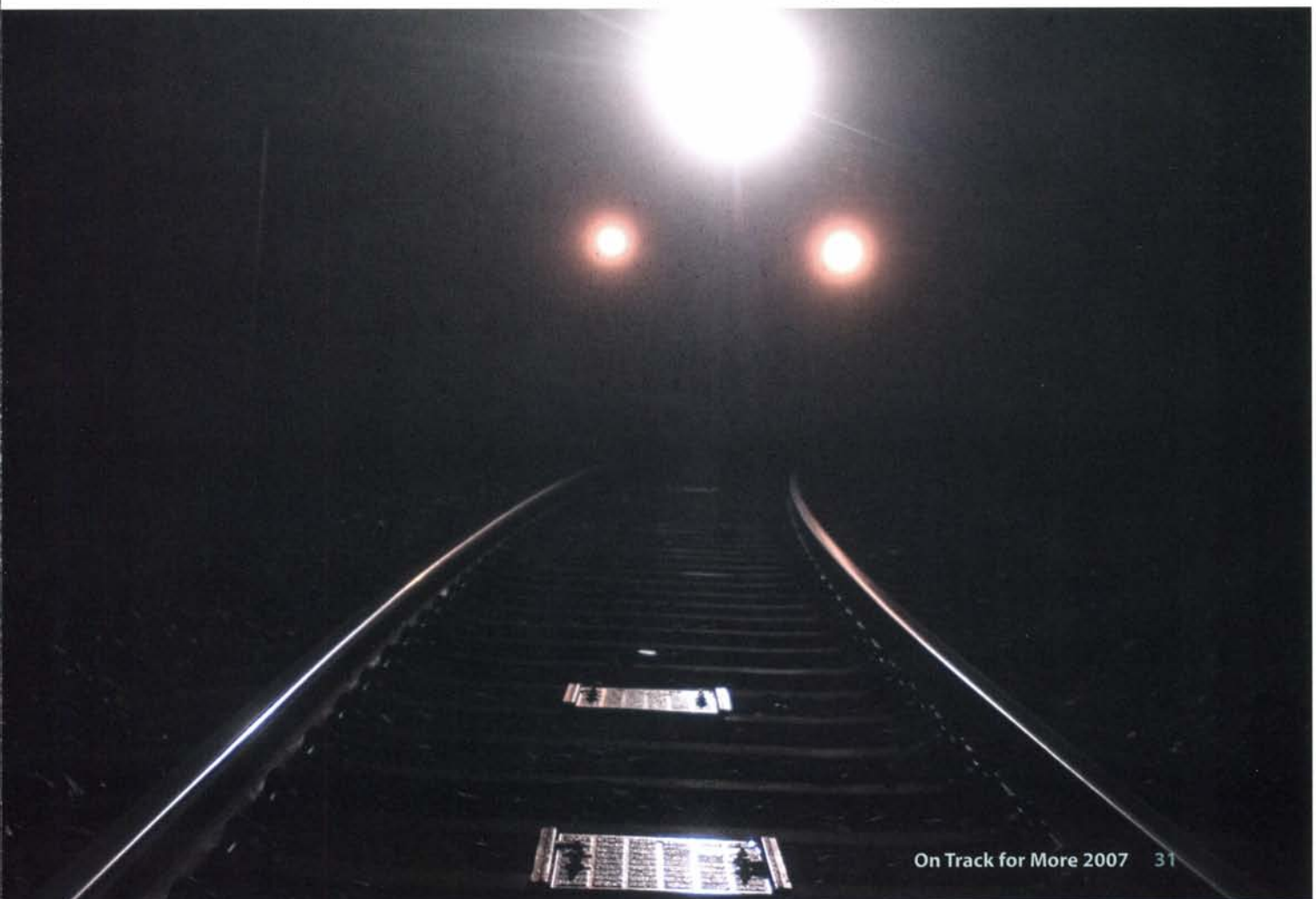
ATC beacons: Mounted on sleepers, these communicate with the train's ATC system and are used in signalling systems to monitor train speeds.
