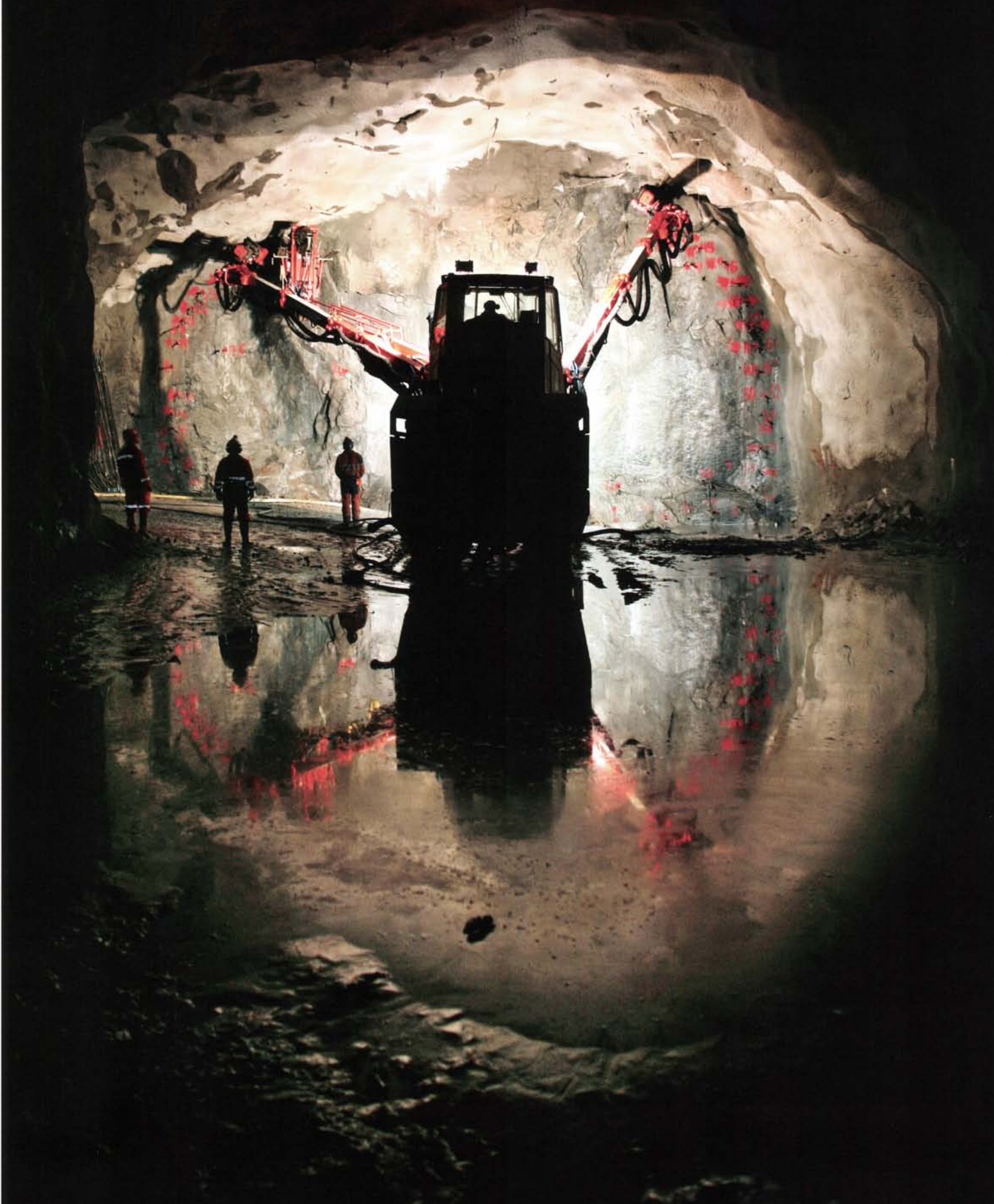
Drilling rig: Ten metres below the gardens of Bærum, the last part of the Lysaker–Sandvika double-track tunnel is being bored.
