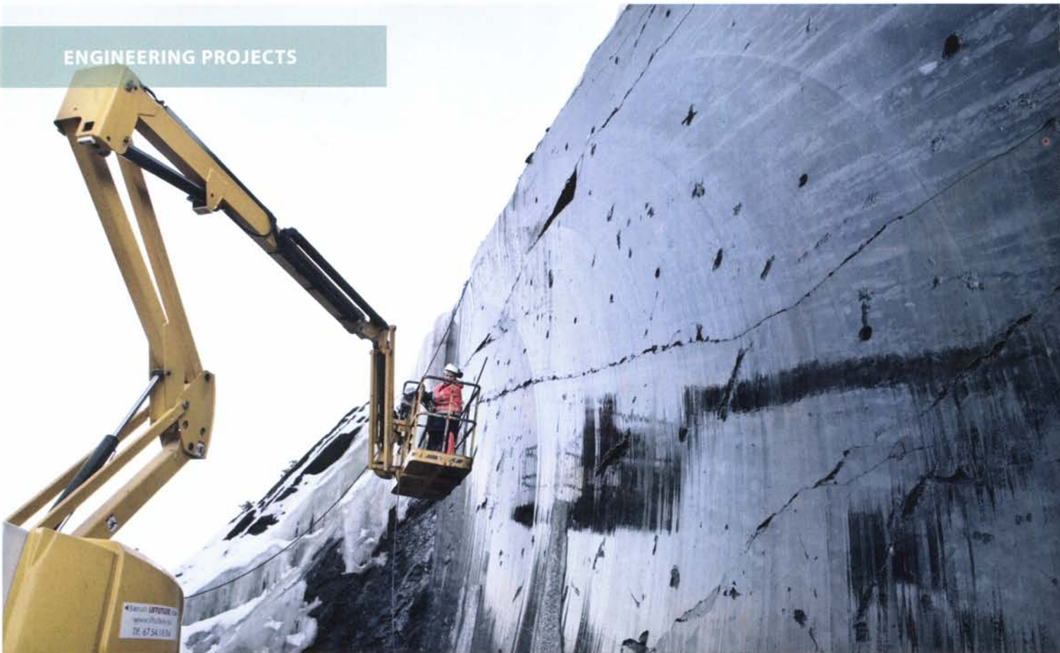
Firmly anchored: Ice is scraped away to find anchor points for the bolts securing the rock cutting alongside Engervannet lake in Bærum.
