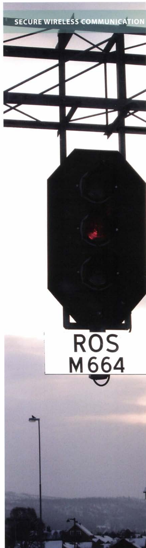
Colour-light signal with location code: 4 400 colour-light signals on the network will be dispensed with when ERTMS takes over.
