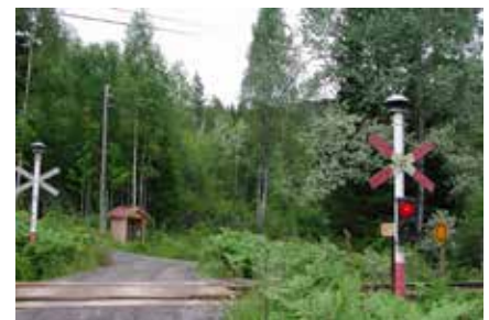
Veisignalanlegg / Warning lights
