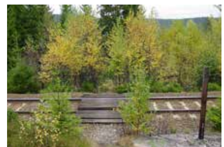
Usikret planovergang / Open crossing
