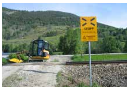
Grind / Level crossing gate
